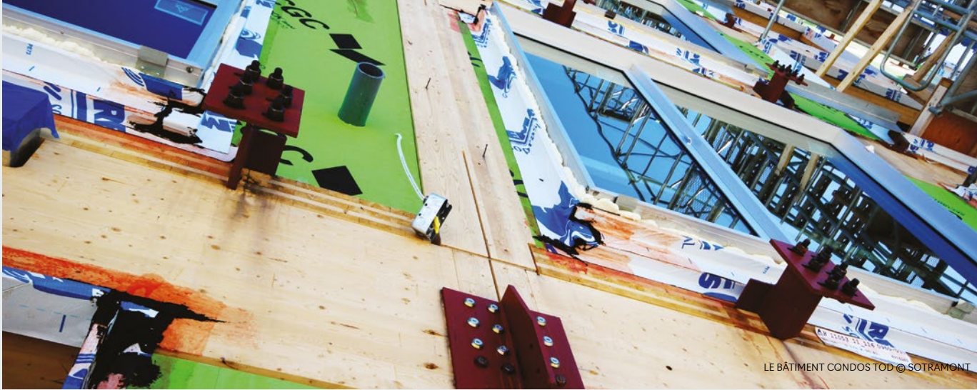
VIEW OF A CLT INTERIOR LOAD-BEARING WALL
